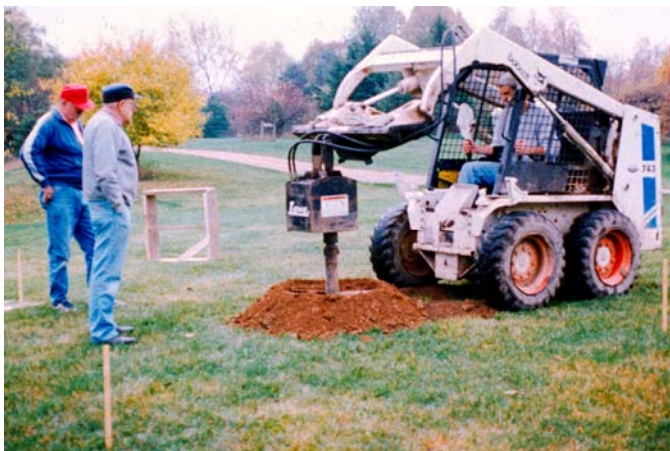
Groundbreaking for Owl Observatory at the Kalamazoo Nature Center. Taken on October 16, 1996.
